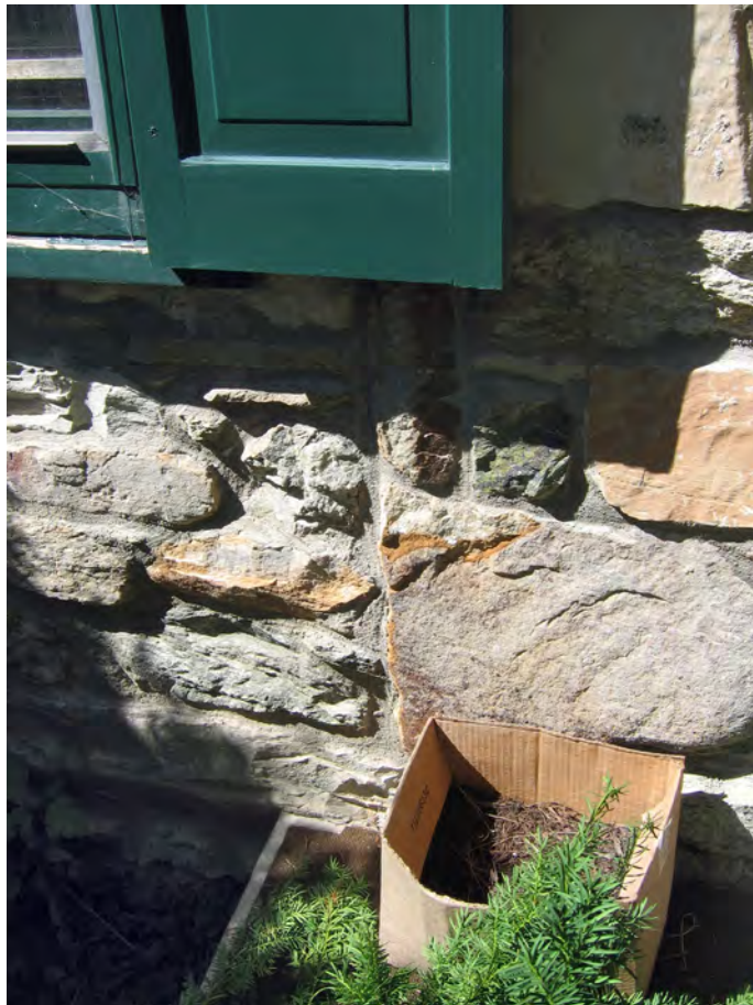
Plate 7: Seam in wall, southern façade.
