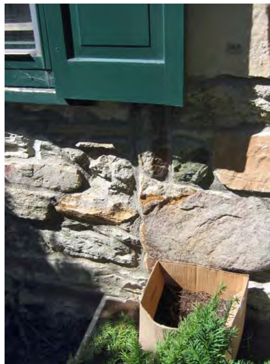
Plate 7: Seam in wall, southern façade.
