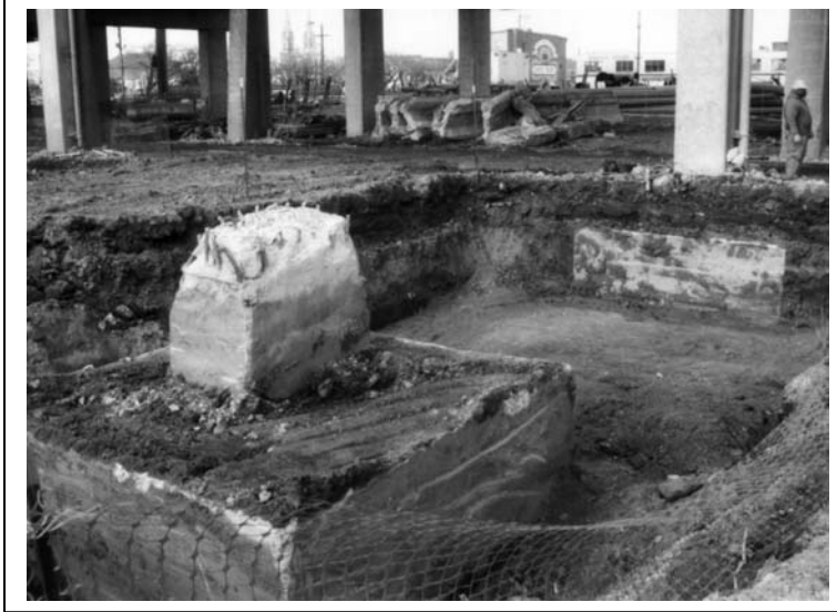
I-95 Reconstruction Project, Philadelphia, Pennsylvania. This project entailed archaeological monitoring during the removal of piers supporting Interstate 95 through the City of Philadelphia and during foundation excavation. Working with construction crews allowed for several features to be identified and avoided. Information concerning the historical development and use of fill material was documented.
